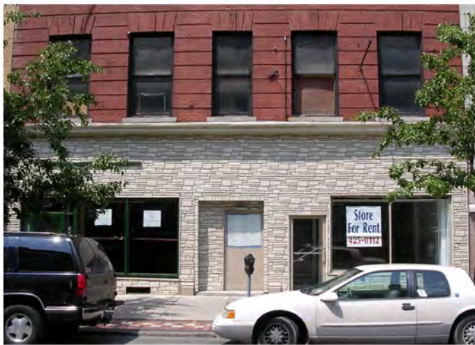
Inappropriate facade treatments of structures detract from the overall character of the building.
